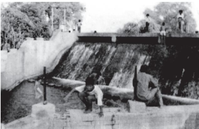
Photo 11.2 Water overflow from the conduit carrying freshwater to the Bhagirathi Water Treatment Plant
