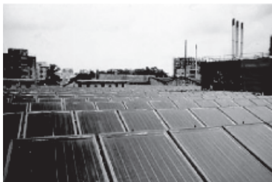
Photo 2.5 Solar power generation
