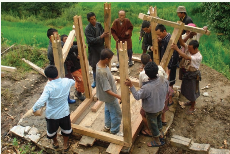
Figure 2 Community members at work constructing a toilet after a workshop Phurpa Thinley, LNW Consulting
