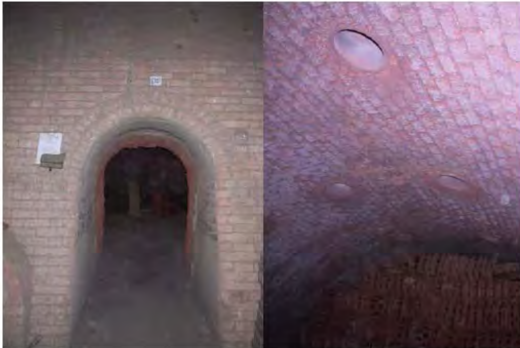
Figure 11: The entrance to one of the chambers in the Hoffmann kiln at Uganda Clays can be seen to the left. The right picture is showing the wholes in the ceiling of the kiln used to feed coffee husks into the kiln.
