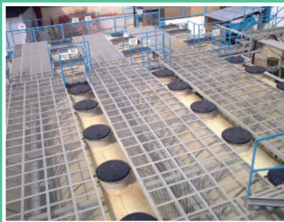
Paco Sewage Treatment Plant Technology: Johkasou - moving bed biofilm reactor
